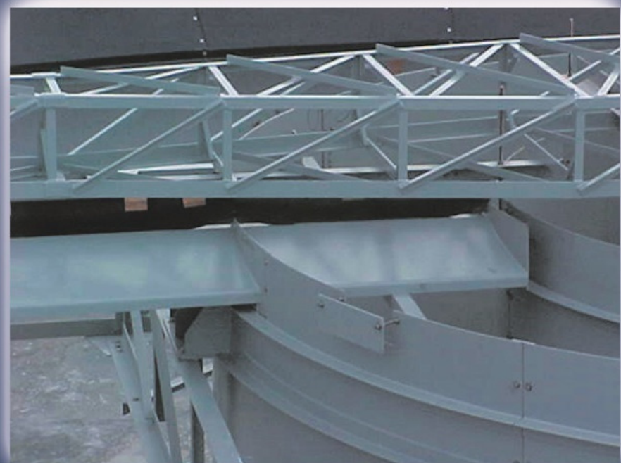
WELL PENETRATING FULL-RADIUS SCUM TROUGHS "Cleans both outside AND inside the well - a feature operators love!"
